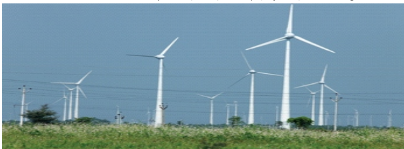
40 MW wind farm in Rajasthan, Source: mnre.gov.in
