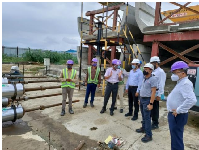
Photo 3: The Afcons engineers demonstrating the pre-stressing procedure at Kanpur metro project casting yard
