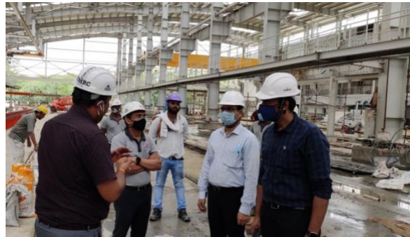
Photo 7: Er. Rishi Gangwar, Chief Engineer (Civil Works) (First from Left) explaining the ongoing work to the envoy with Project Director, Er. Arvind Singh (Second from Left)
